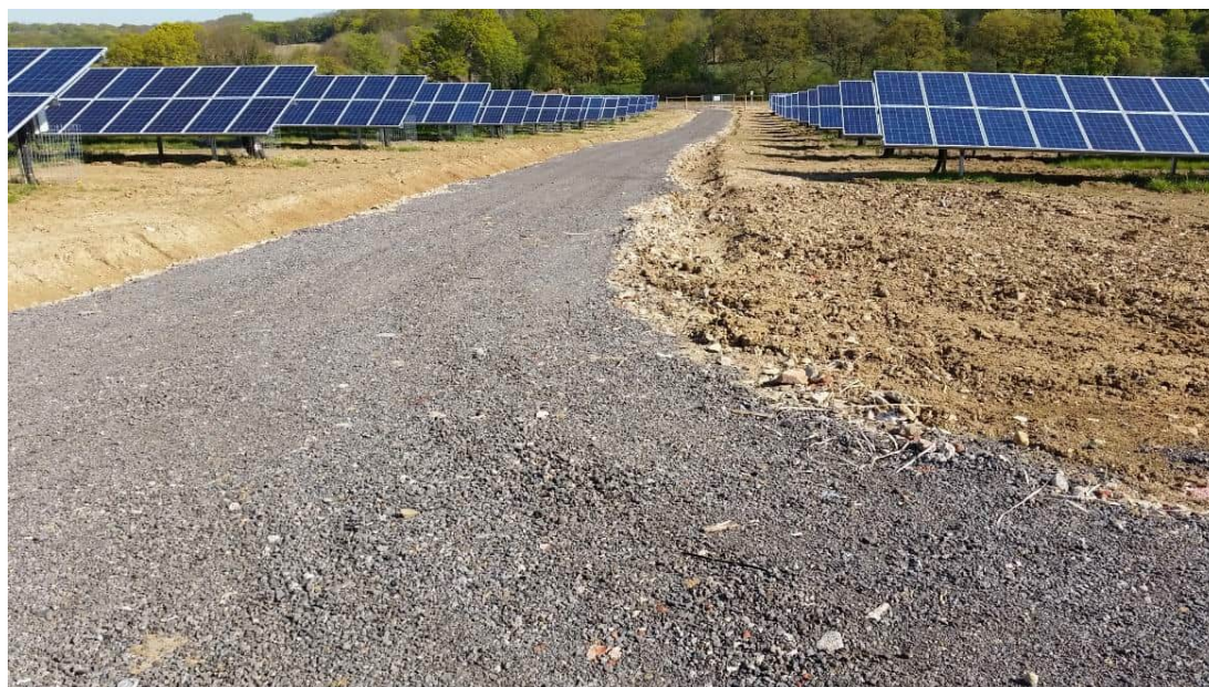
Plate 8. Typical crushed stone access track laid on hardcore and geotextile (photo during construction phase and prior to landscaping)
