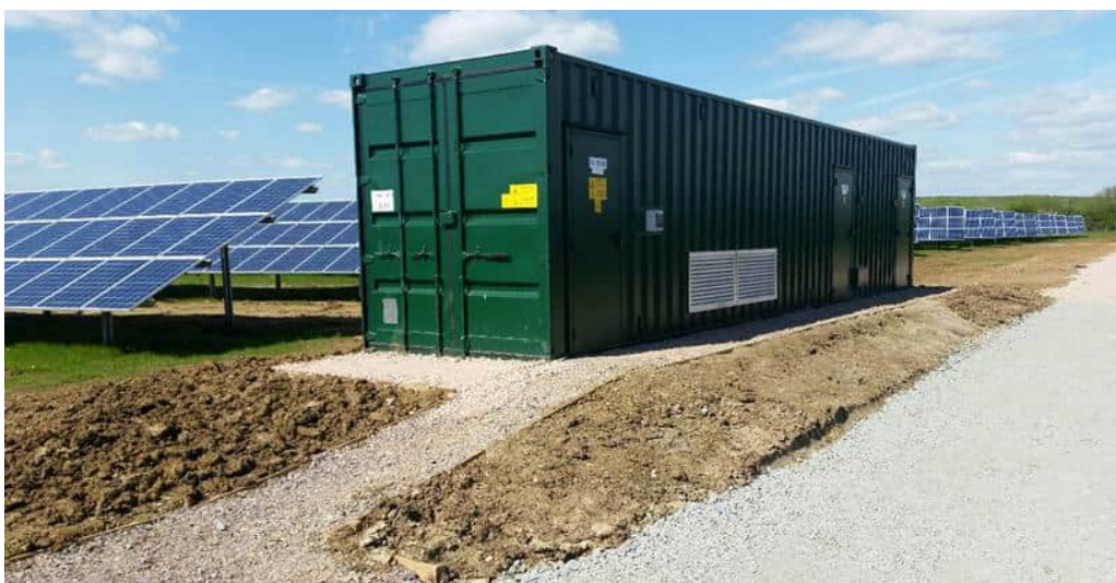
Plate 6. Typical unit housing the transformers and switchgear
