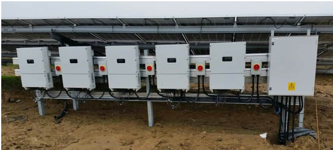
Plate 4. Typical string inverter installed next to PV modules
