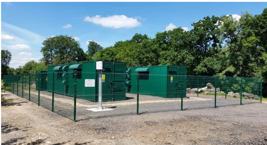
Plate 5. Typical pair of central inverters
